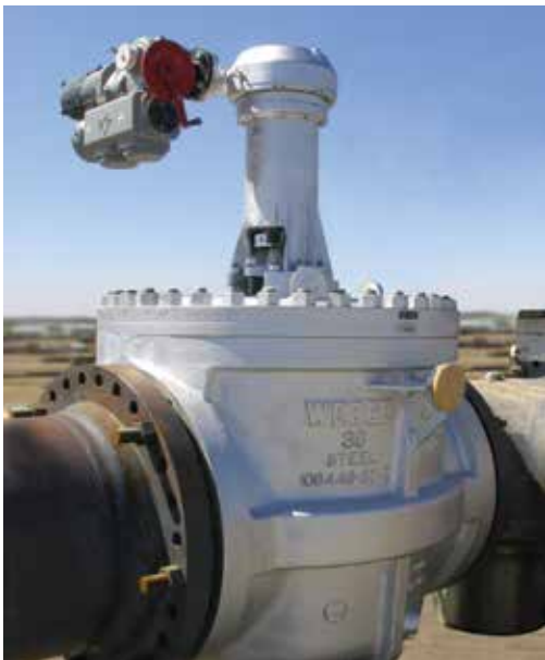
WEDGEPLUG™ installation at Suncor Millennium 2 Coker project, Fort McMurray, Alberta Canada. Electrically actuated 30" full port WEDGEPLUG™, overhead vapor line isolation service.
