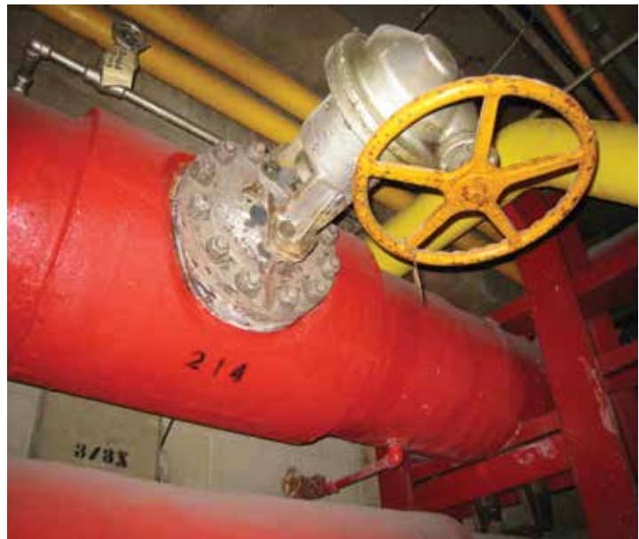
WEDGEPLUG™ installation at Chicago's O'Hare Airport. O-ring style plug used to supply water to the airport and also used in hot water loop to melt ice on runways.
